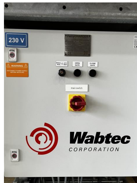
3261 – Control Panel on socket
