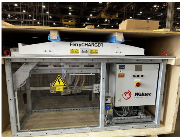
3258 – Charging Socket for the shoreside charger
