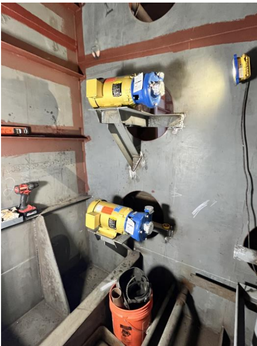
5645 – Propulsion Cooling Motors in Engine Room
