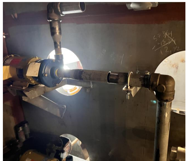
5716 – Propulsion Cooling System Piping and Pump
