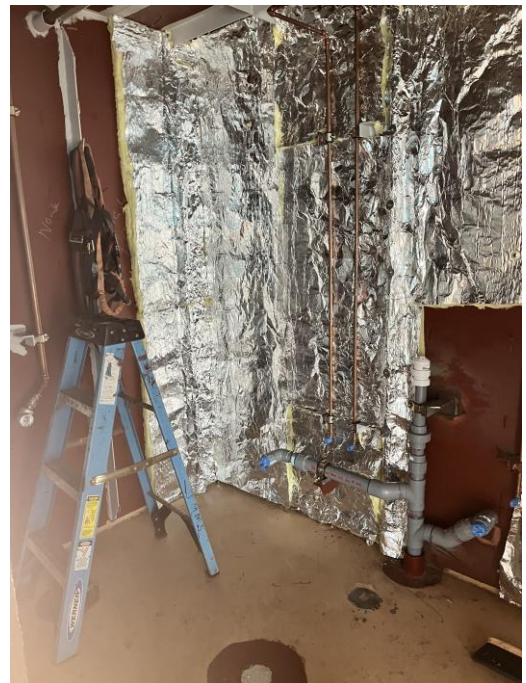
5745 – Insulation in Crew Restroom on 02 Deck
