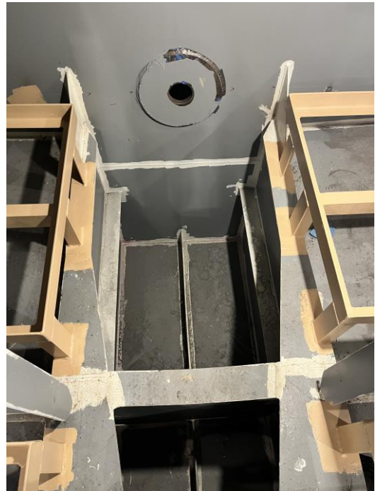
5750 – Shaft Line in Void 2
