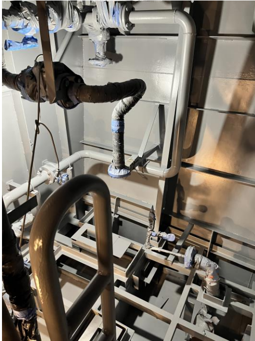
5746 – Paint Behind Engine Room Stairs
