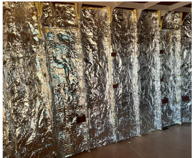
5743 – Insulation in Elec Room below Pilot House
