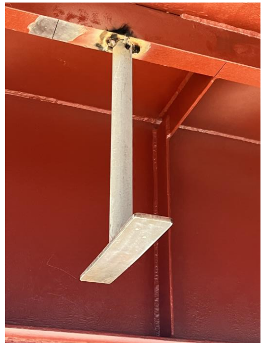
5466 – Typical Light Support Installed
