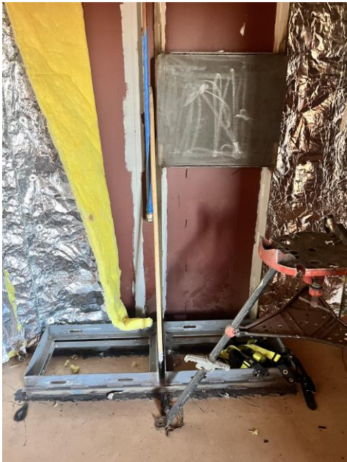
5742 – AC Elec Panel Foundation in Elec Rm Below Pilot House
