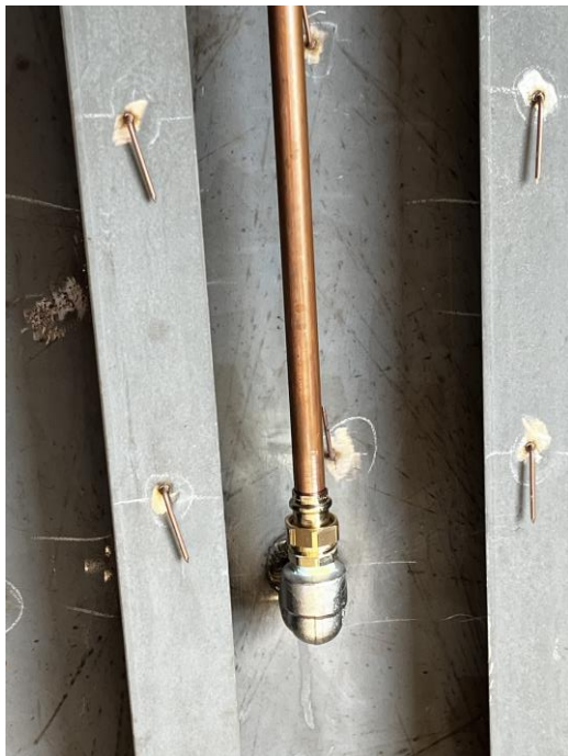
4348 – Potable Water Piping
