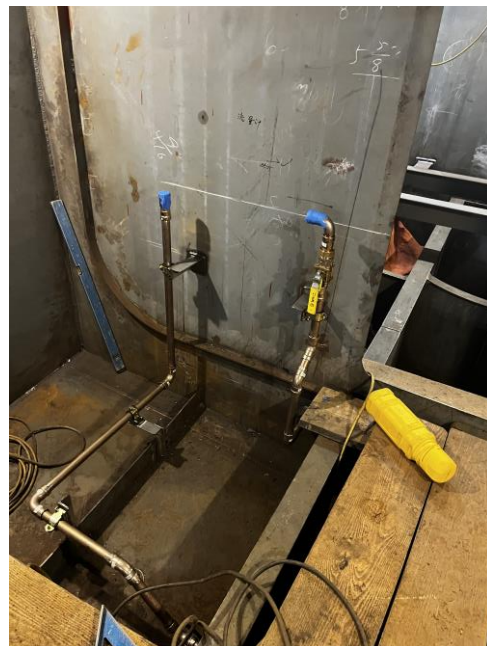
4392 – Potable Water Piping(left) and Propulsion Cooling Piping (right) w/Shutoff
