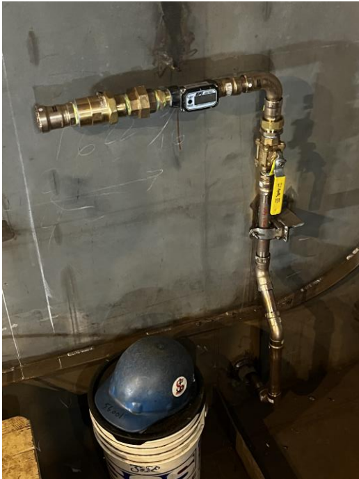
4214 – Potable Water Line in Engine Room
