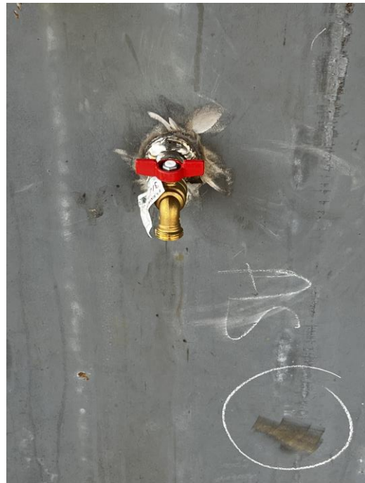
4347 – Potable Water Spicket – Main Deck
