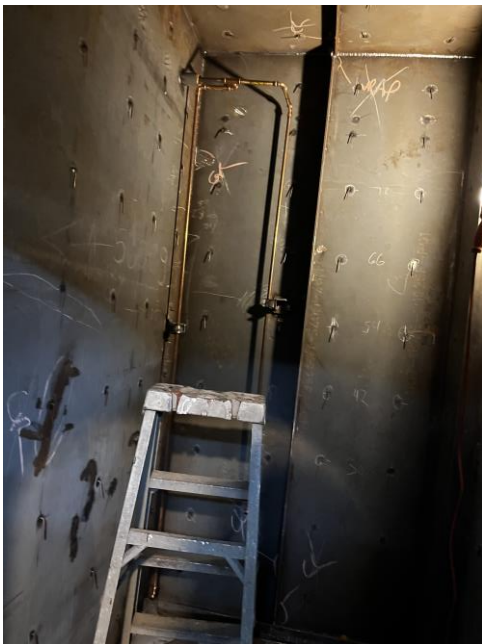
4370 – Potable Water Piping in 02 Bathroom with Bulkhead Penetrations
