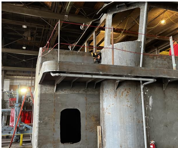
4290 – Drain Piping Around Pilot House
