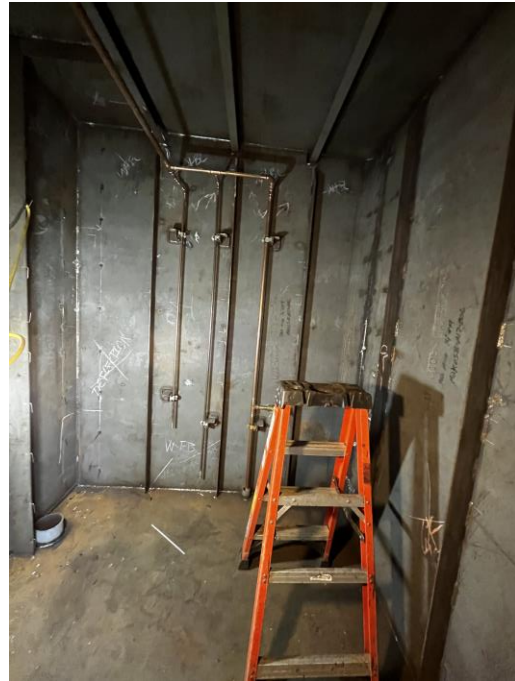
4390 – Potable Piping Installed in a Bathroom
