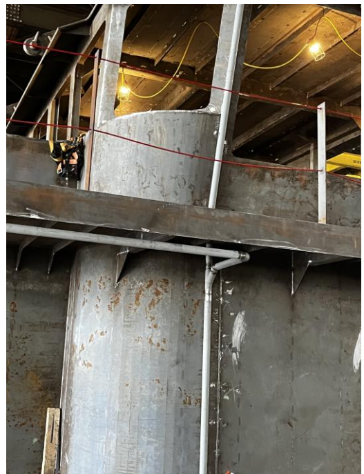
4289 – Drain Piping Around Pilot House
