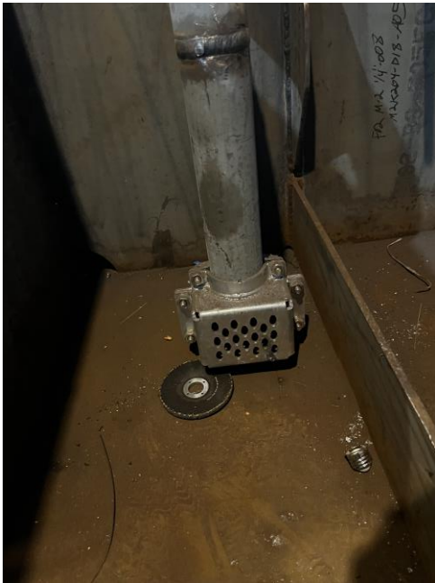
4412 – Strainer for Bilge Piping in Switchboard Room
