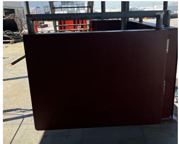
4487 – Typical Swing Gate at Man Overboard Station
