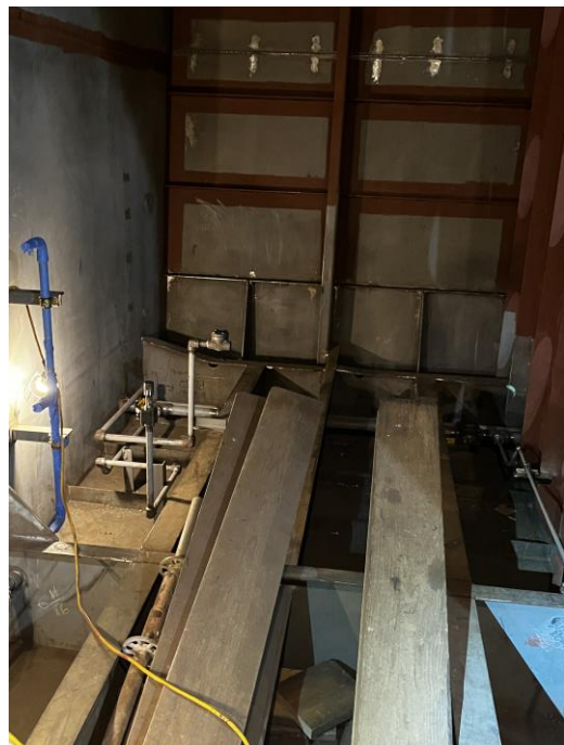
4648 – Piping in Engine Room
