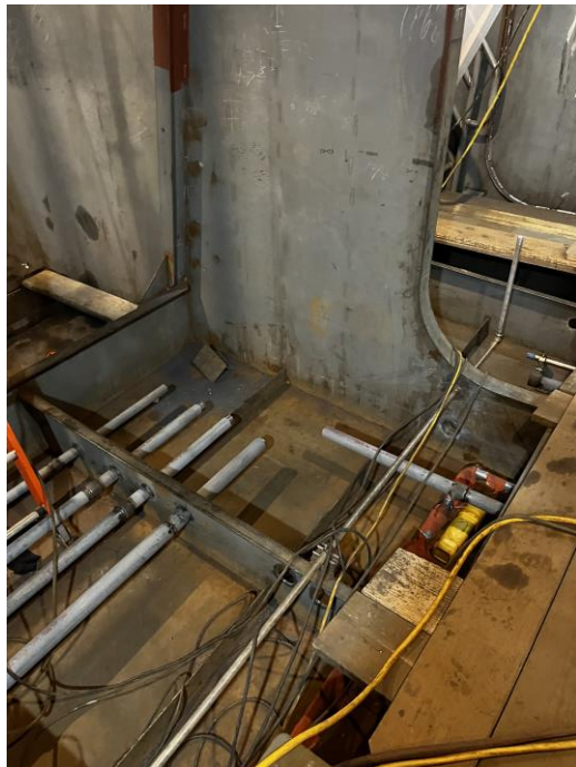
4575 – Piping in Engine Room
