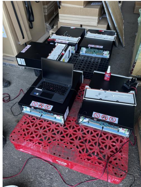
4693 – Checking State of Charge for Sample of Battery Modules
