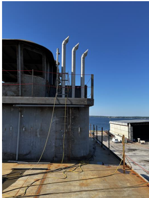
4563 – Last Exhaust Stack Added, for Furnace
