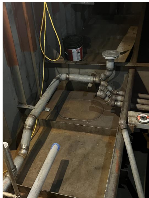
4688 – Piping Manifold Area
