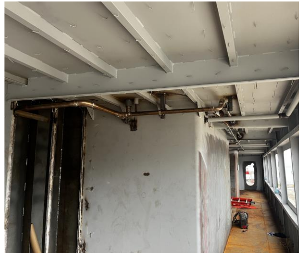
4763 – Piping in 01 Deck Starboard Cabin
