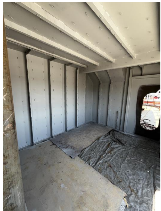
4507 – Paint Coat in Main Deck Starboard Cabin
