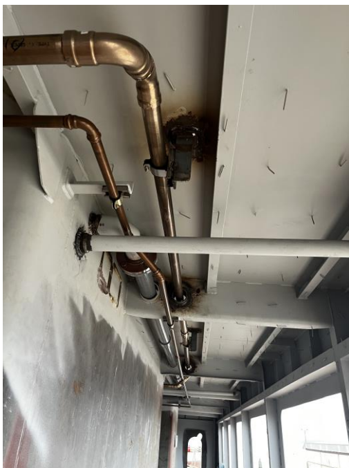
4764 – Piping in 01 Deck Starboard Cabin
