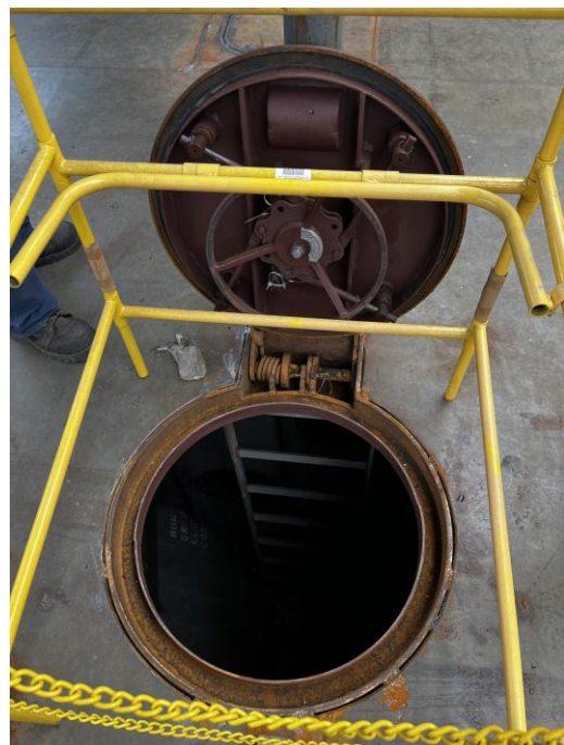
4752 – Hatch with Ladder to Engine Room Below
