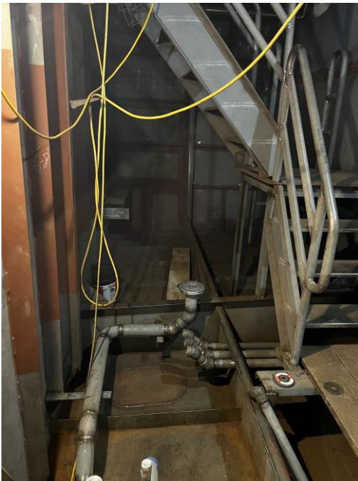
4679 – Piping @ Engine Room Stairs
