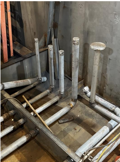
4623 – Piping in Engine Room
