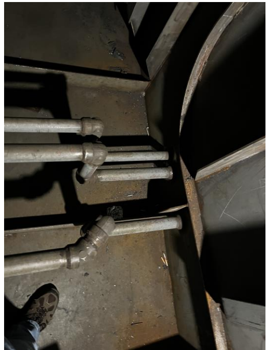
4505 – Piping in Engine Room
