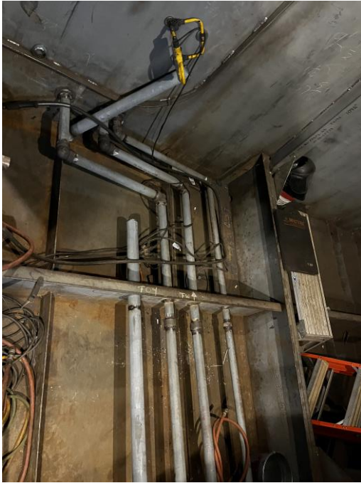
4571 – Piping in Engine Room
