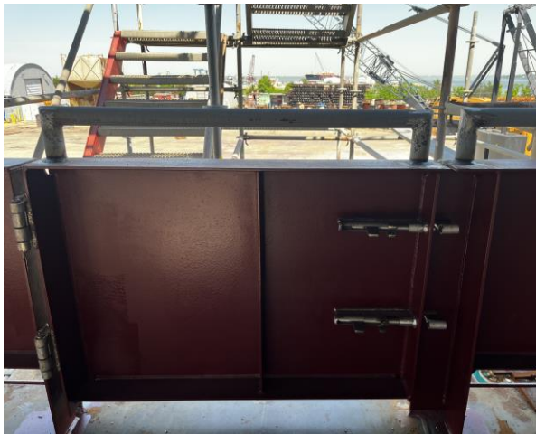
4485 – Typical Swing Gate at Man Overboard Station
