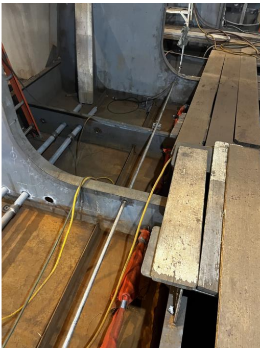
4506 – Piping in Engine Room
